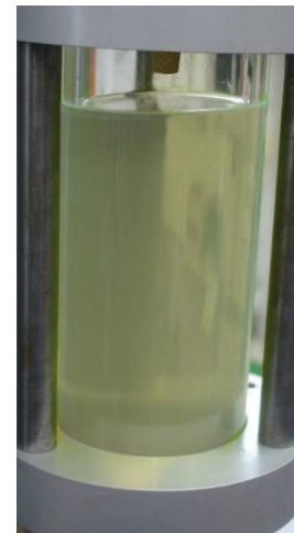
Fouled refrigerant, compressor faulty.
